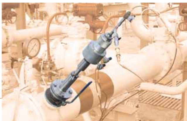
In-Line Installed probe. Sonda installata in linea.
